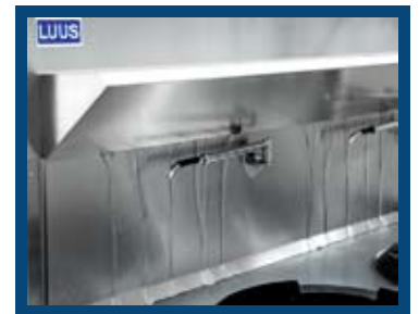
Water Cooling System
